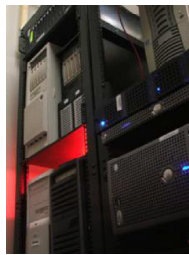
Web Server Racks
